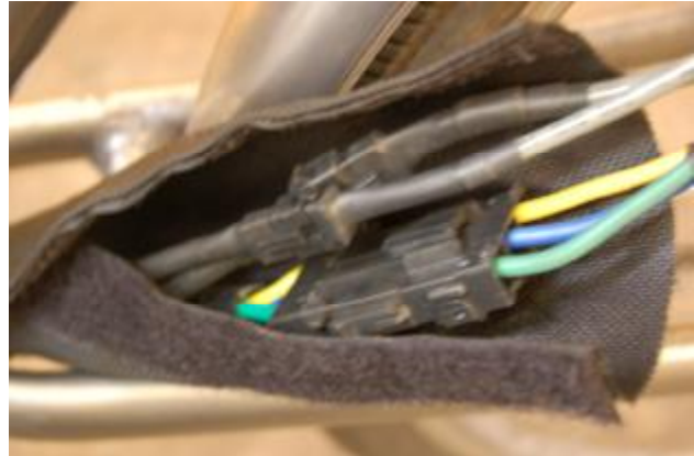
(20) Cables Connectors Wrapped in Op-
